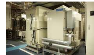
JIZAI HEAT installed at the Rinkai Factory
