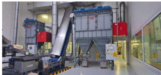
Dust collector installed at a food factory in Mexico
