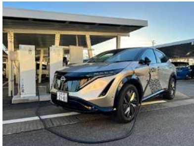
EV and charger/discharger installed at Matsumoto Precision Inc.
